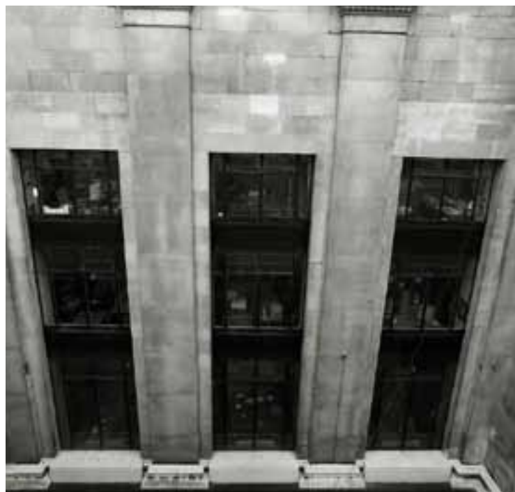
Full-length window openings from the 1930s. Only recently closed up, it is proposed to reuse these openings in the building to form the doorways through to the galleries and new centre.
